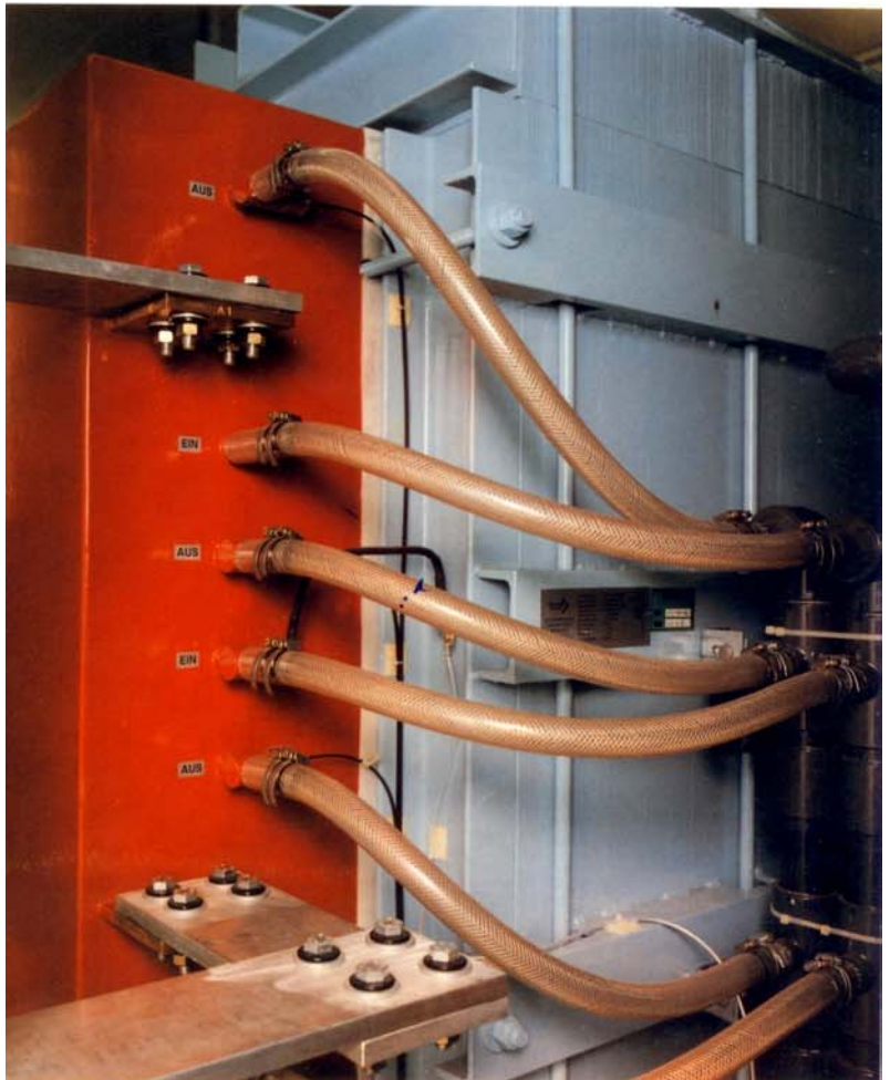
Water cooled smoothing reactors in the intermediate DC circuit. The electrical connections are the massive copper bars. The reactors are cooled by water hoses.
