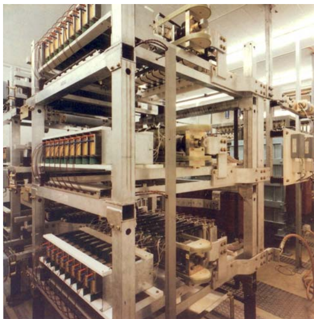
Our picture shows part of the line inverter, particularly the three racks of the power electronic frame work. On the lefthand front side the electronic controls of the thyristors can be seen. On the right side the extrarapid fuse of the DC intermediate circuit can be seen. Befour that two ignition sets for the extrarapid fuses
